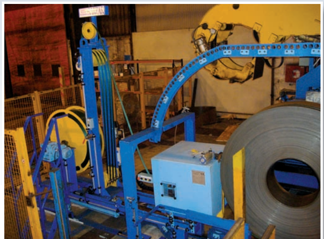
Strapping machine with horizontal head for the circumferential strapping of coils with polyester strap, situated in the pickling line.
